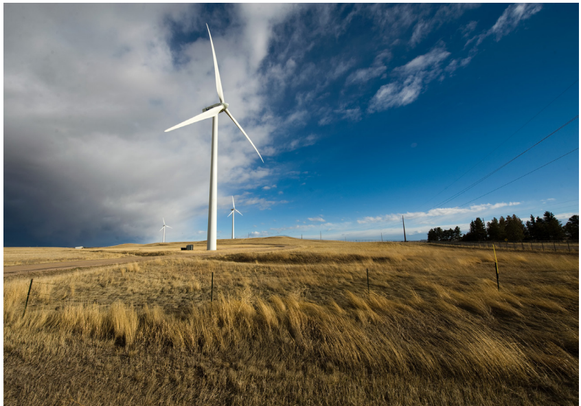
Wind turbines at Warren Air Force Base, Wyoming face the wind coming across the high plains, providing electrical energy that goes directly into the base power grid.
