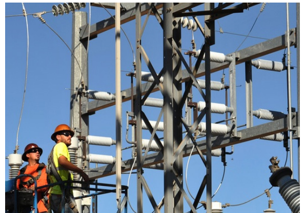
Figure 1. Contractors work on electrical substation renovations at Beale Air Force Base in California. Photo by: Airman 1st Class Tristan Viglianco, 9th Reconnaissance Wing Public Affairs.
